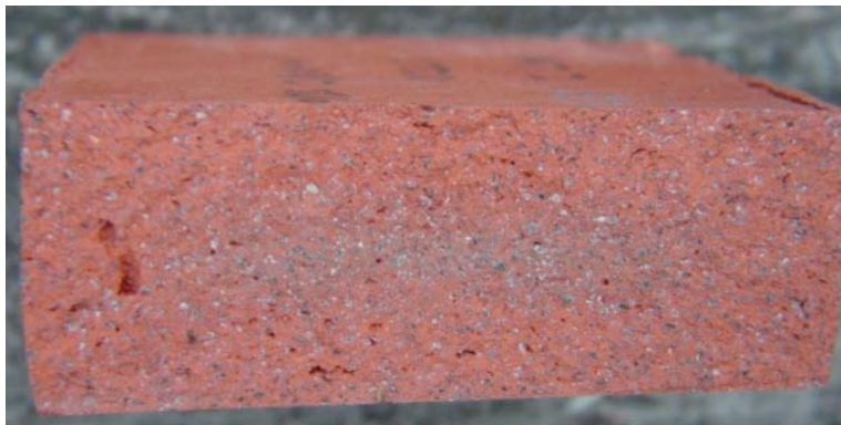
Broken brick face
